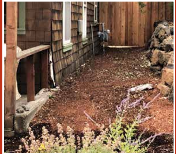
Bark mulch against combustible wooden siding is a flammable situation.
